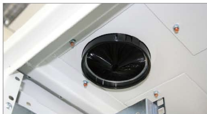
Example of installed plates and cable opening in a rack
